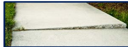
Typical Trip Hazard
