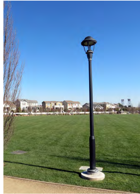
Example of Neighborhood Park Lighting
