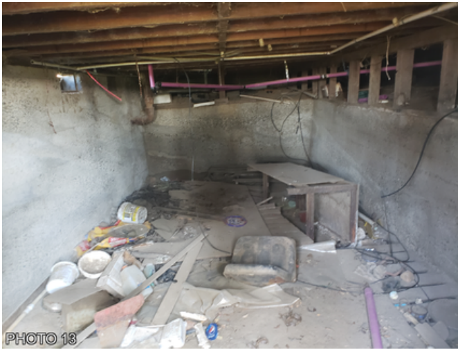
PHOTO 13 BASEMENT OF HOME OFF PARADISE ROAD
