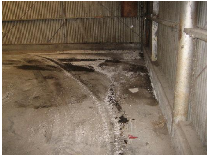
STAINED CONCRETE INSIDE THE BARN
