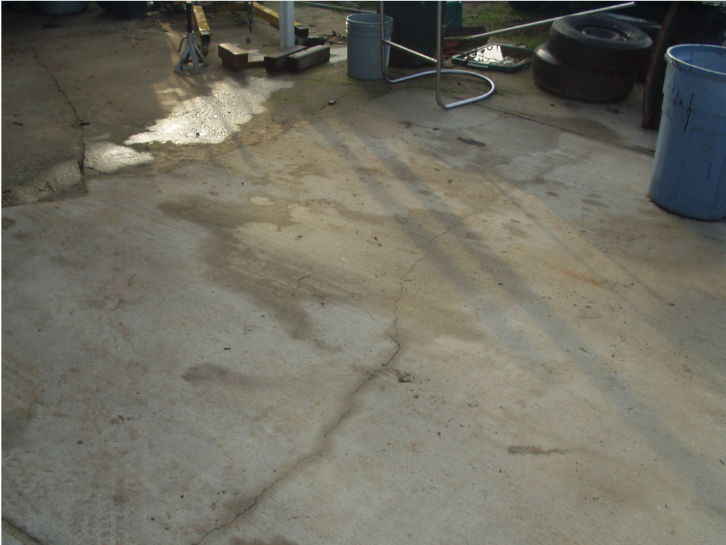
Concrete stain next to workshop entrance. View to SE.
