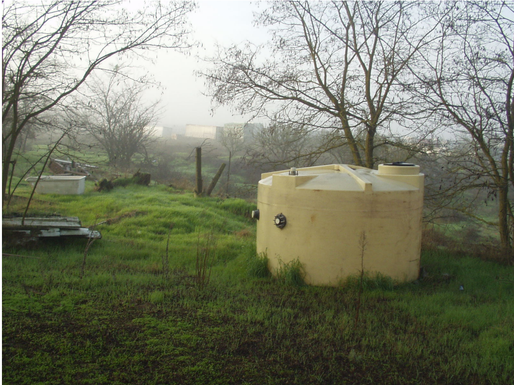
Above ground water storage tank. View to SW.
