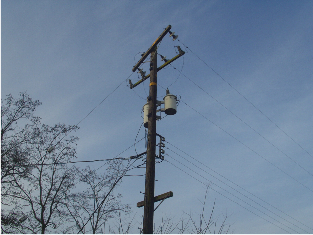
Pole mounted transformers located west of Residence #1. View to SW.
