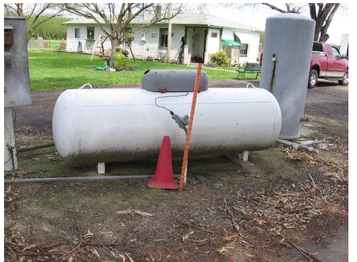
PROPANE TANK ON CONCRETE STRIPS
