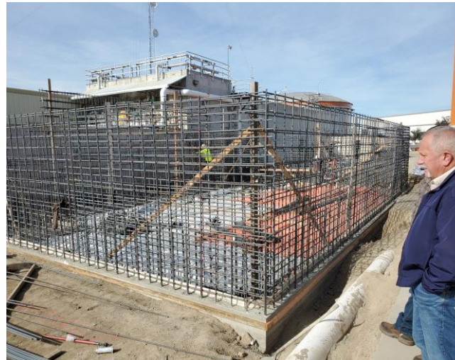
Waste Water Treatment Facility
