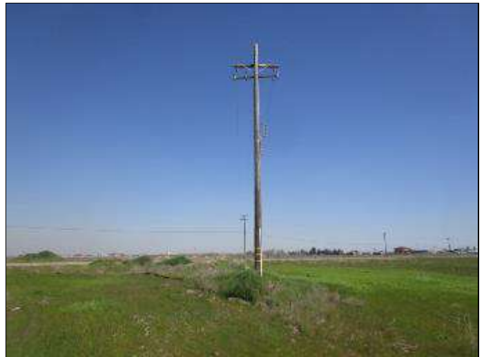
10. Power pole at the northern end of Parcel 192-020-600
