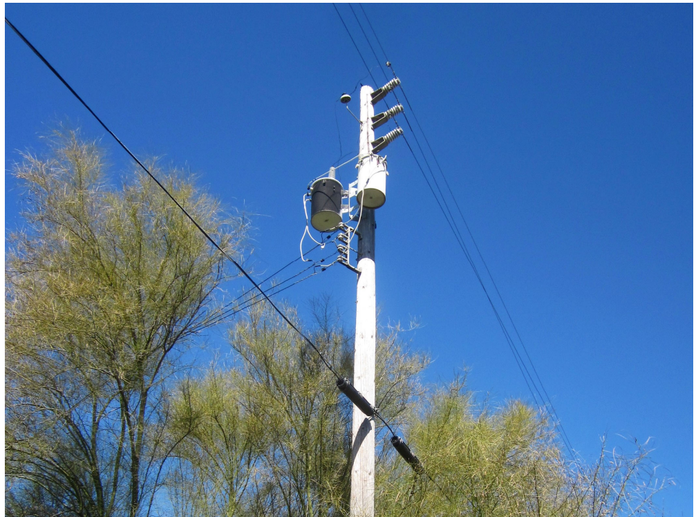
Photo 6: View of the pole-mounted transformer adjacent to the west of Manthey Road.
