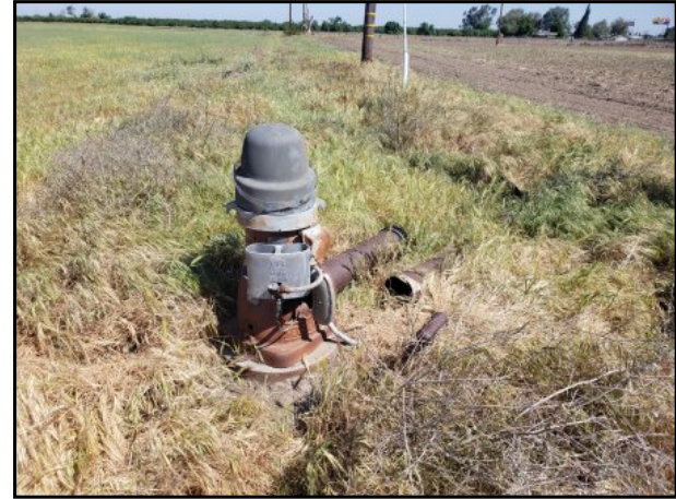
14 : Photograph of abandoned water well located in southeast corner of subject property.
