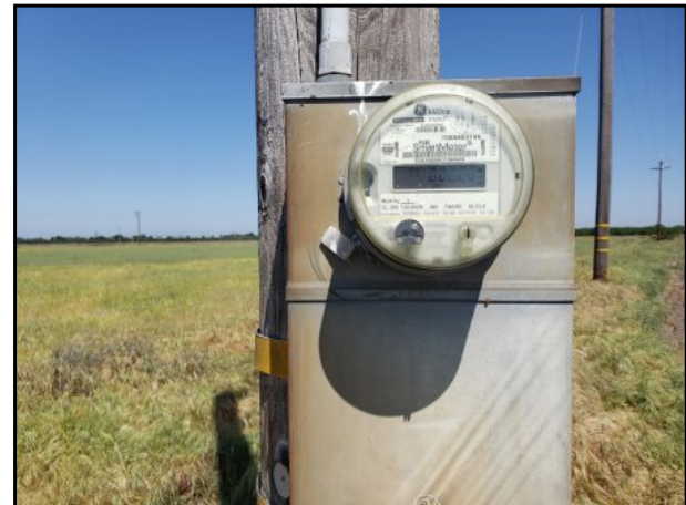
16 : Photograph of electric service to abandoned water well located in southeast corner of subject property.
