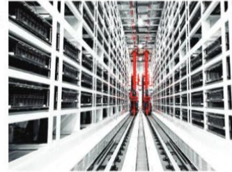
Tesla opened another California facility, a utility scale battery manufacturing plant to produce the company's largest energy storage unit — the Megapack. Photo courtesy of Tesla, Inc.
