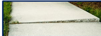
Typical Trip Hazard
