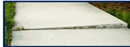
Typical Trip Hazard
