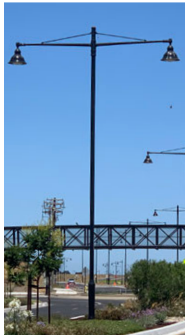
Arterial Street Lights
