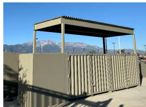
Photo Example 8 Enclosed refuse areas
