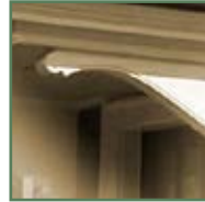
Corbel to fascia
