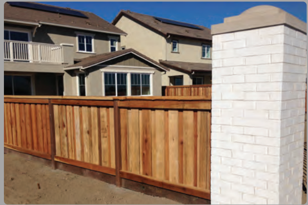
8' Tall Masonry Column with 5' Lake Front Transition Fence
