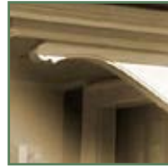
Corbel to fascia
