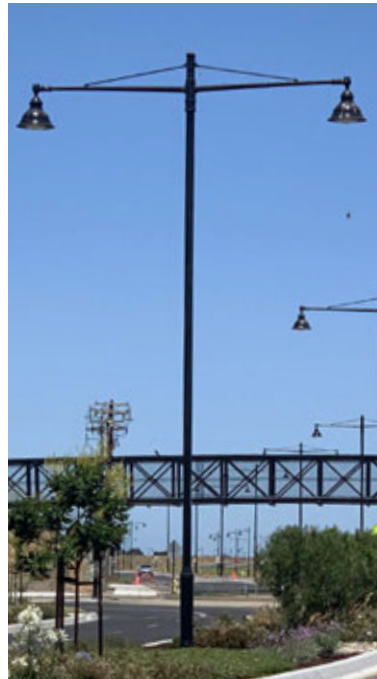
Arterial Street Lights
