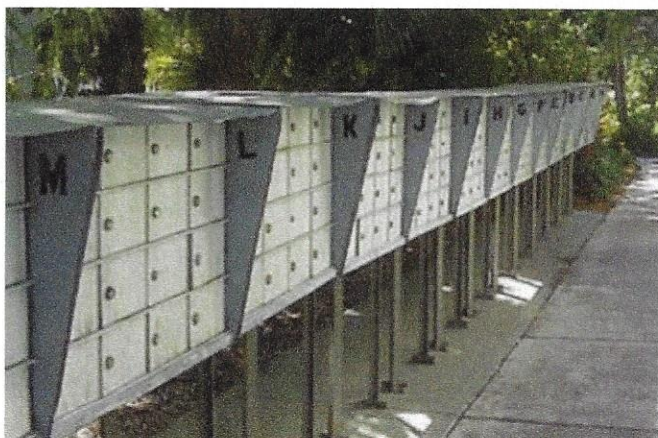
Obsolete NDCBUs are no longer permitted for replacement or new installations.
