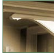
Corbel to fascia
