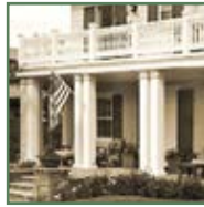
Double wide wood posts
