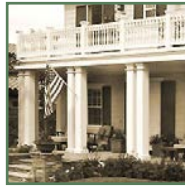
Double wide wood posts
