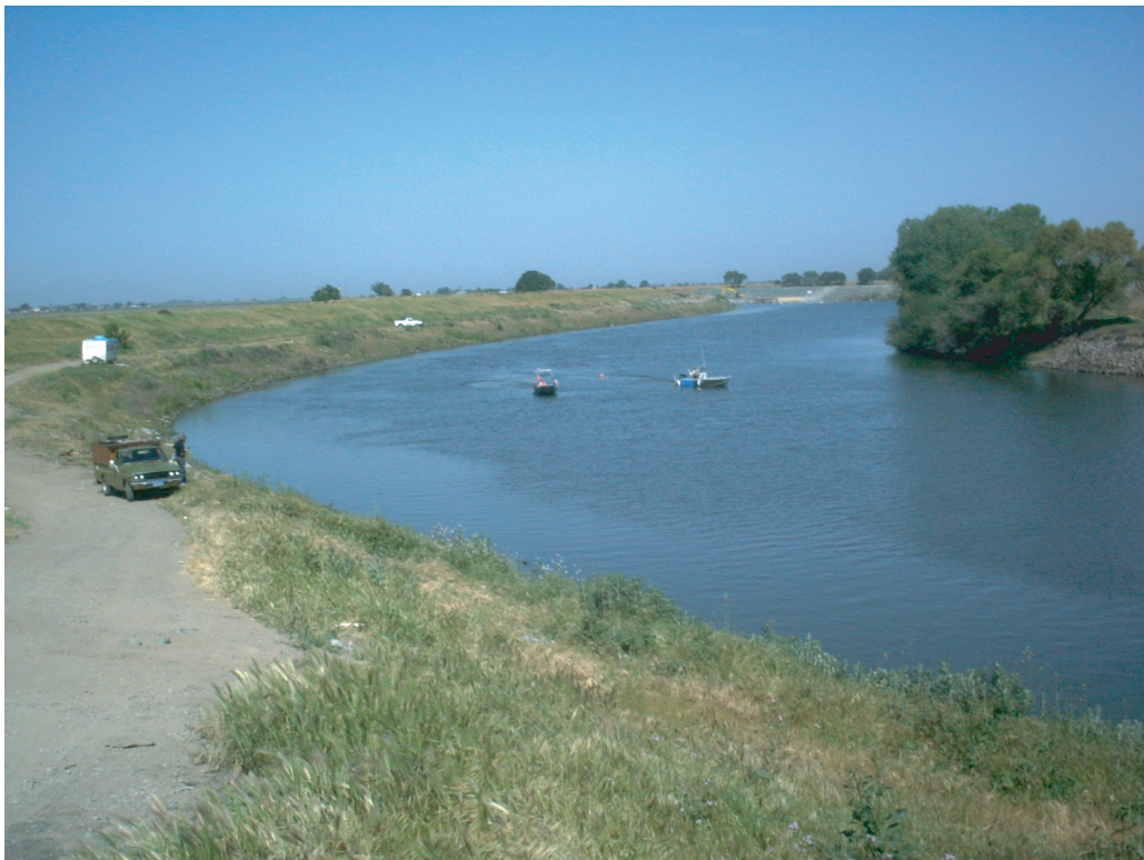
Viewpoint 4: San Joaquin River levee face, head of Old River in background
