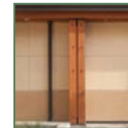
Column with exposed bolts
